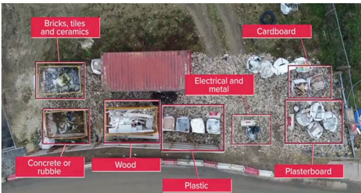
Aerial shot of the project plot waste area from Langley Grange in Yorkshire
