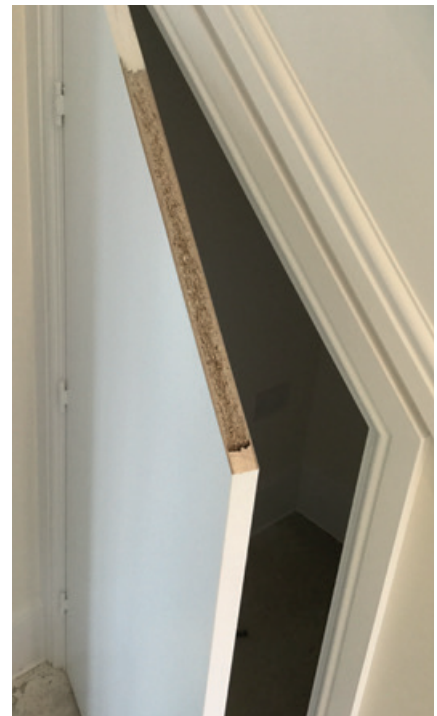
D06 Door under stairs of Oxford was chipped during installation
